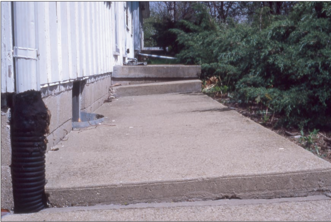
Figure 24 A moat-type depression along the foundation wall and lowered sidewalk and patio slabs caused by the kind of peripheral drainage system shown in figure 23.
