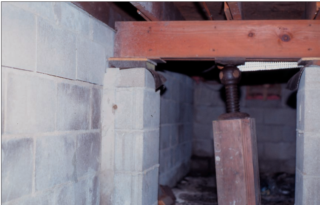
Figure 25 This main beam is not attached directly to the foundation wall. Because the beam is settling a different amount than the foundation and because some of the thick layers of shims are compressing, cracks have developed in the house above the beam.
