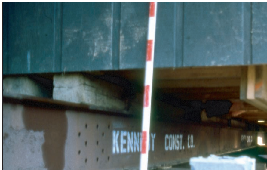
Figure 17 Concrete blocks of a crawl space have been removed to make room to jack the house to a level position. I-beams support the re-leveled house.
