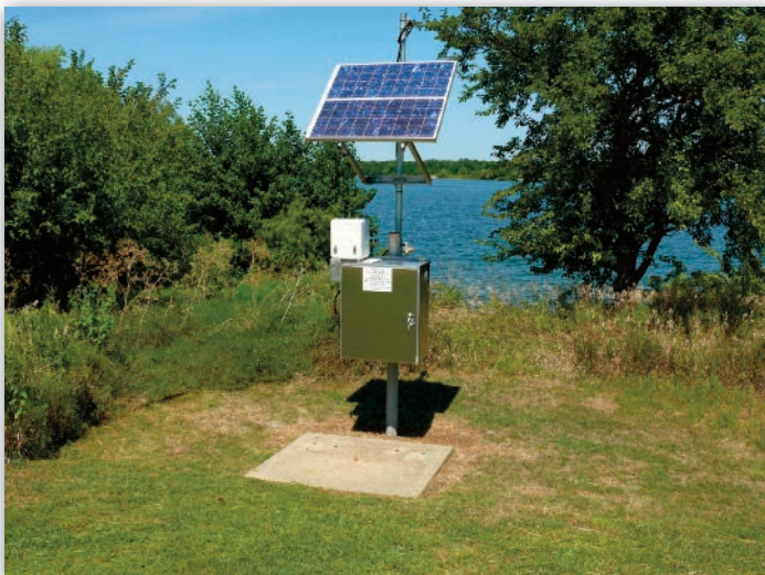
Sixteen GDN detectors surround each nuclear power plant to monitor gamma radiation in the environment.
